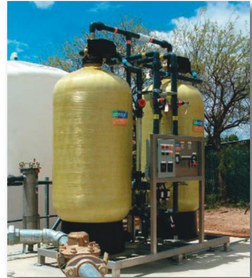
Arsenic Removal - Rimrock, AZ
